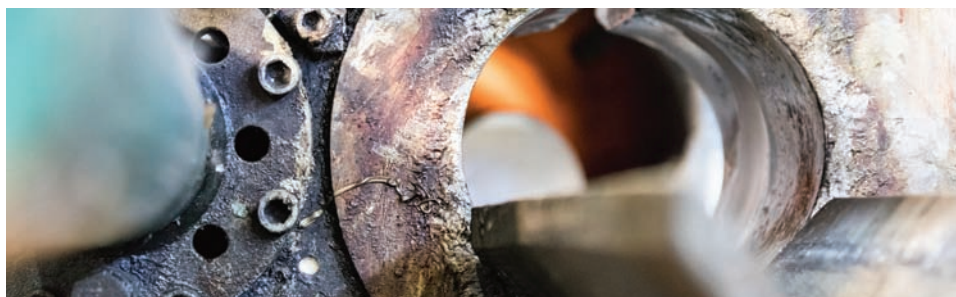
HAZARDOUS EXSH1 SPOT HOUSING
